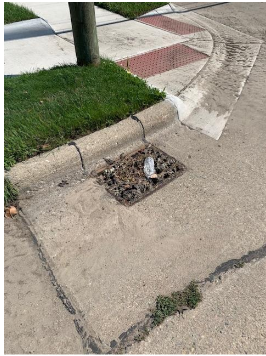
Post Storm - Debris, Dirt, Litter
