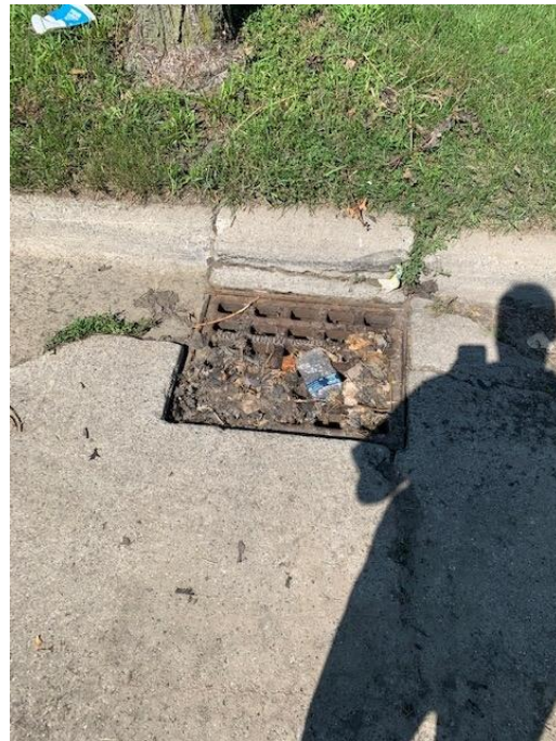
Post Storm - Debris & Litter
